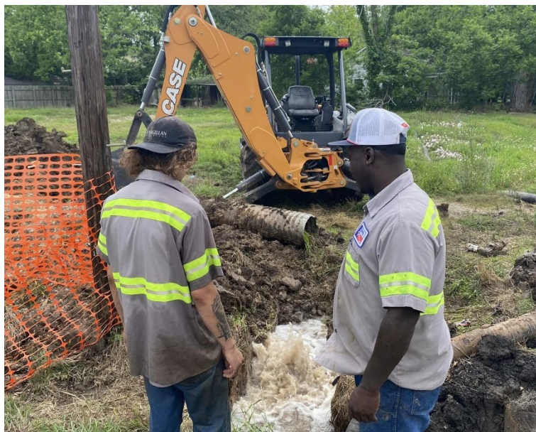
Public Works employees uncover a major leak at 2nd & Orange Streets.
